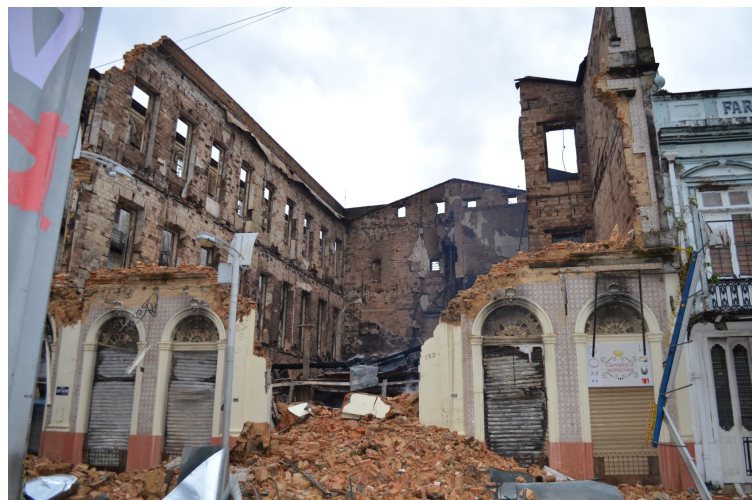
Fig. 1: An example of challenges that restoration architects find in cultural buildings. Case of the fire followed by Casa Carvalhaes collapse, in Belém historical center, that co LACORE voluntary action to collect integrated cultural assets from the rubble. Commerce Center, Belém. Source: Thais Sanjad, 2015.
